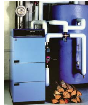
A heat storage system will produce and store hot water throughout the year.
